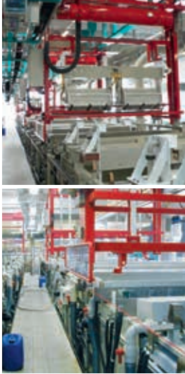
Figure 1: Barrel plating line Figure 2: Rack plating line
