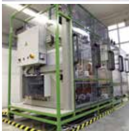
Figure 1: DynaChrome® Plus line showing housing Figure 2: New ion exchange system
